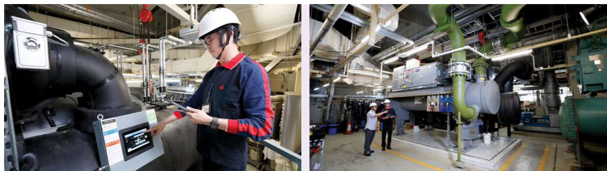
機電署為警察總部更換兩台老化的製冷機組。新機組採用低全球升溫潛能值的雪種，能源效益更高。 The EMSD has replaced two ageing chillers at the Police Headquarters. With the use of low-GWP refrigerants, the new chillers offer enhanced energy efficiency.
