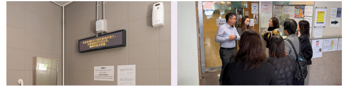
(左)今年，我們陸續為康文署轄下多個康體場地安裝智能意外感應系統，並加設語音辨識求助功能及顯示屏，有助偵測可能發生的意外，並在出現異常情況時即時通知值班人員。 (右)康文署助理署長(康樂事務)1 馮妙玲女士(後排左三)與機電署代表到訪長沙灣體育館。 (Left) We continued to install the Intelligent Fall Detection System in multiple LCSD recreation and sports venues this year. Enhanced with voice recognition and display screens, the system helps detect potential accidents, and promptly alerts duty personnel in case of anomalies. (Right) Ms Fung Miu-ling, Assistant Director (Leisure Services)1 of the LCSD (3rd left, back row), visited Cheung Sha Wan Sports Centre with EMSD representatives.
